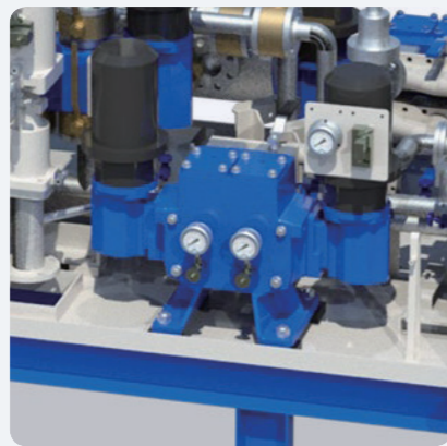
P-01 / 02, P-03 / 04 Supply Pumps, Circ. Pumps
